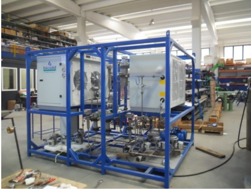
Figure 13: Picture of the Cooling Plant before installation in the pit
